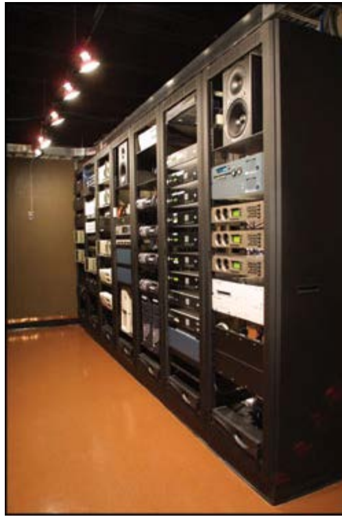
The central rack room is a showcase of its own.
