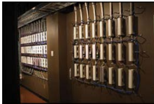
The wiring wall, behind the main racks, uses Krone blocks for the multipair cable terminations.
