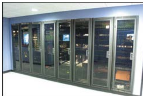
The outer racks face into a common hallway.
